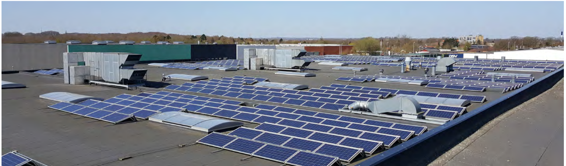
200kW Solar Panels installed at Budweg's Plant in DK
